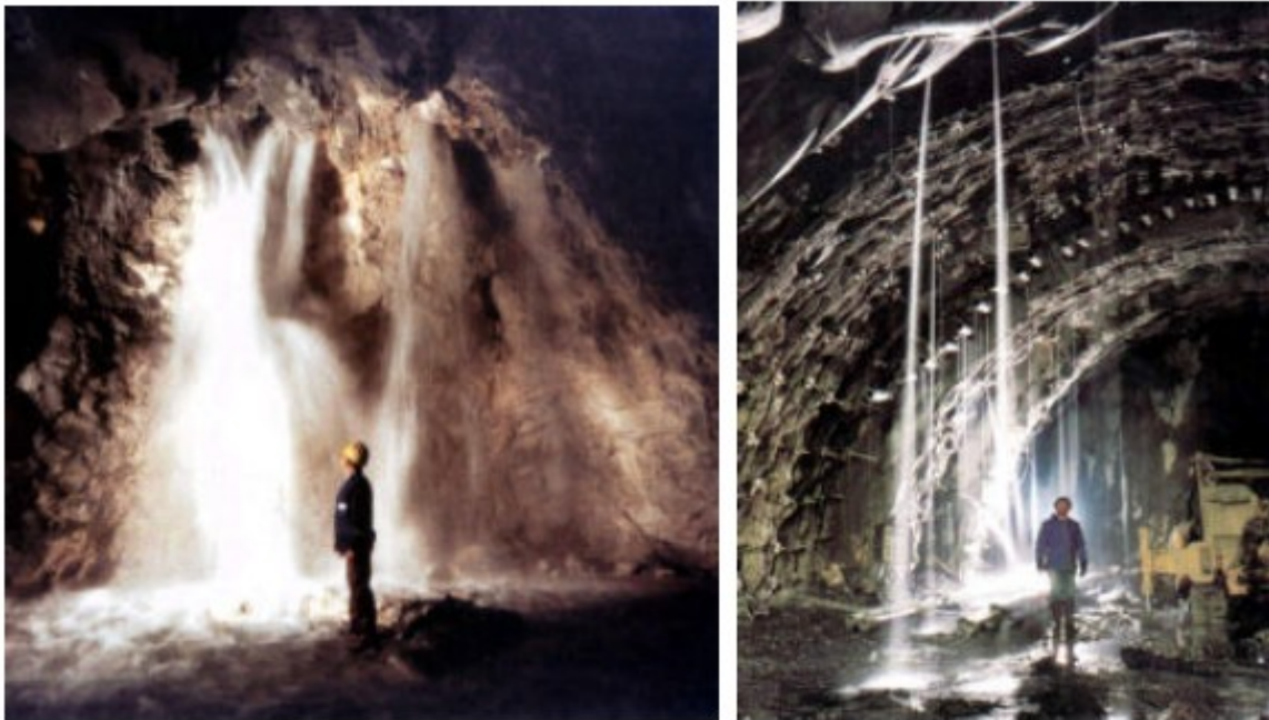
Fig. 5.7 – The effect of interaction of the Serena Tunnel, Railway Line Parma – La Spezia, with the surrounding aquifer (Source: Civita, M.V., 2005).
