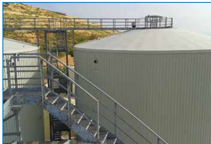
Figura 5 – Malta North Waste Treatment Plant, digestori.
